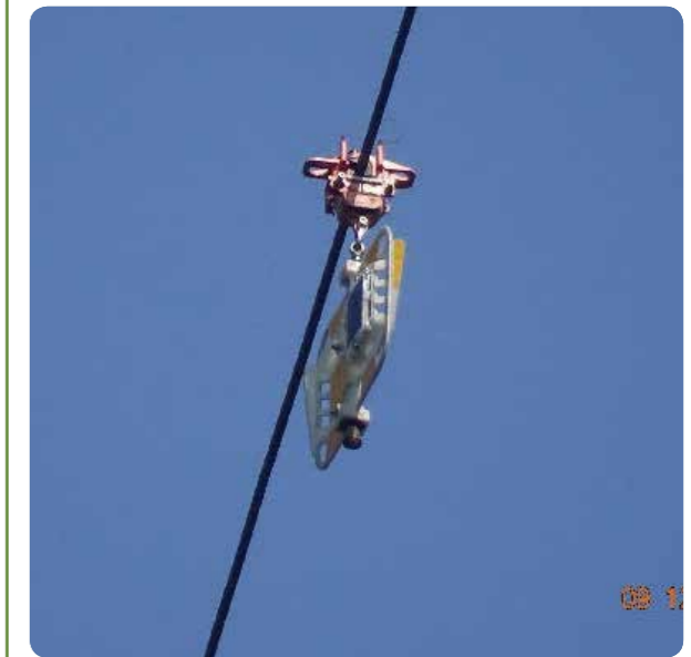
Bird Diverters installed in POWERGRID Transmission Lines for protection of Avifauna
