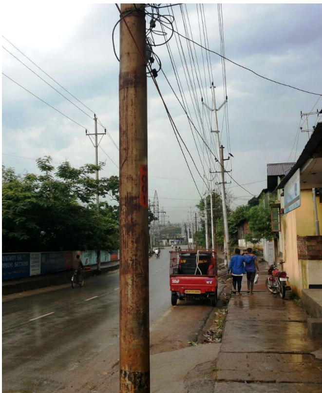
33 kV line inside city area of Assam
