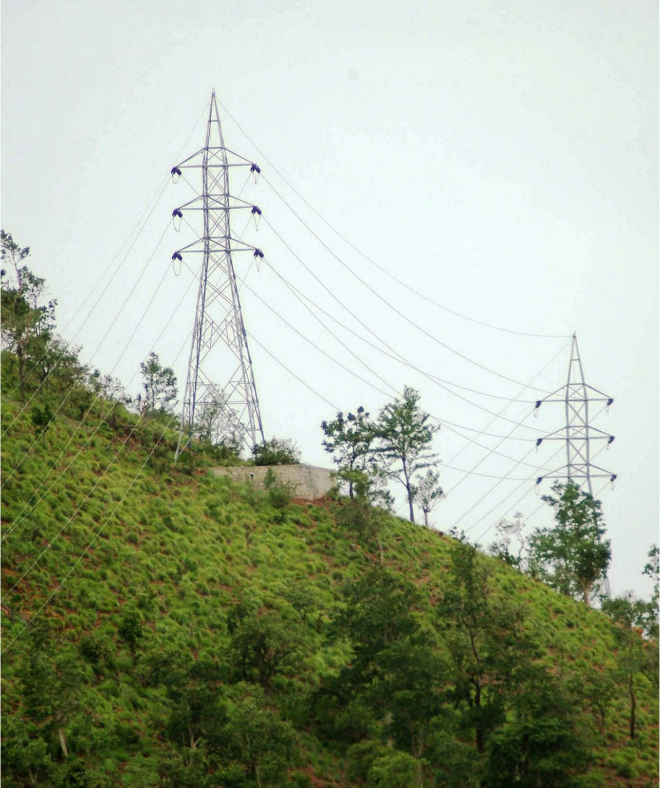
Fig. -1 132 kV line depicting actual position along with RoW and extent of damage
