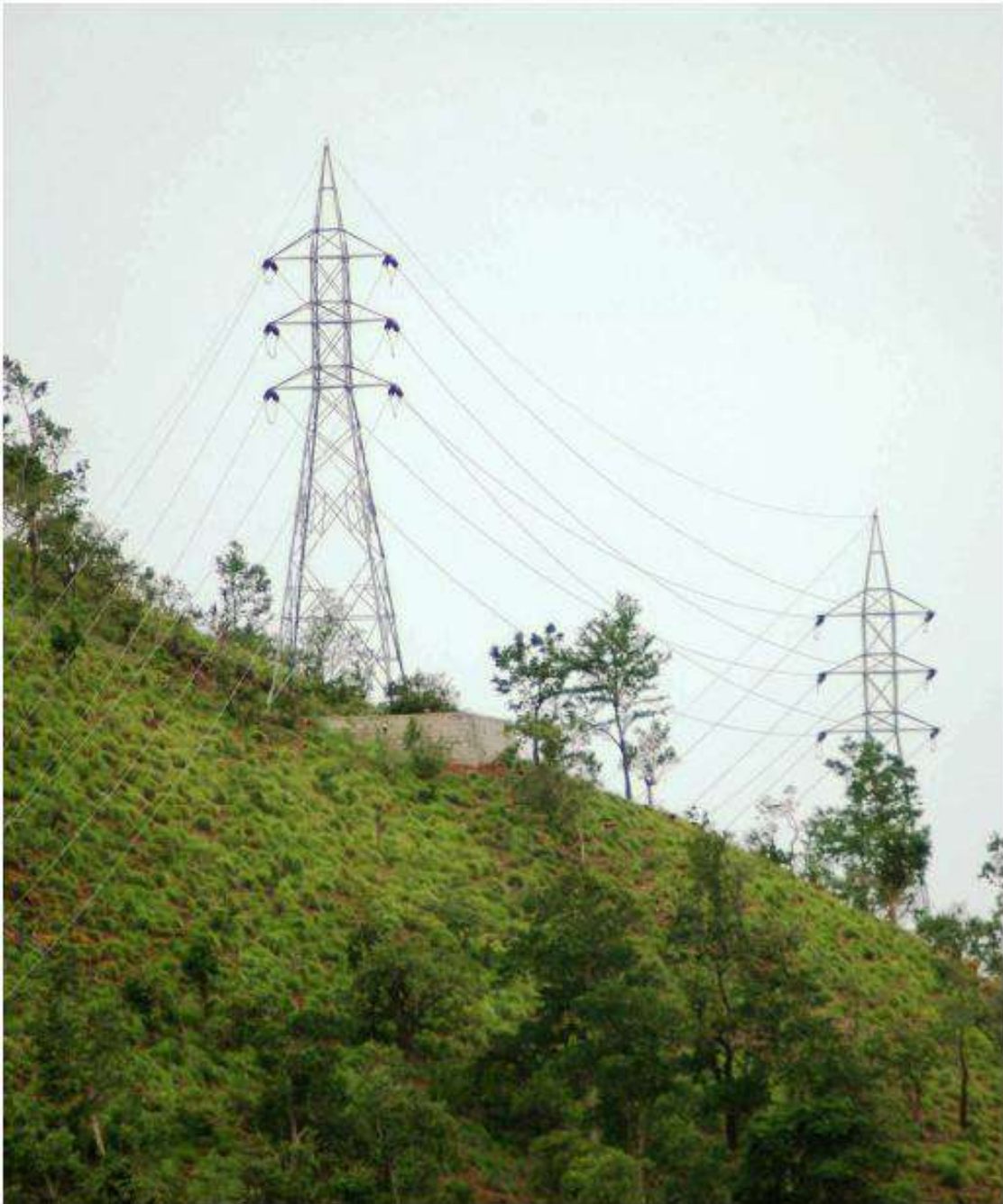
Figure 5-3: 132 kV TL depicting actual position along with RoW in Undulating terrain and extent of damage
