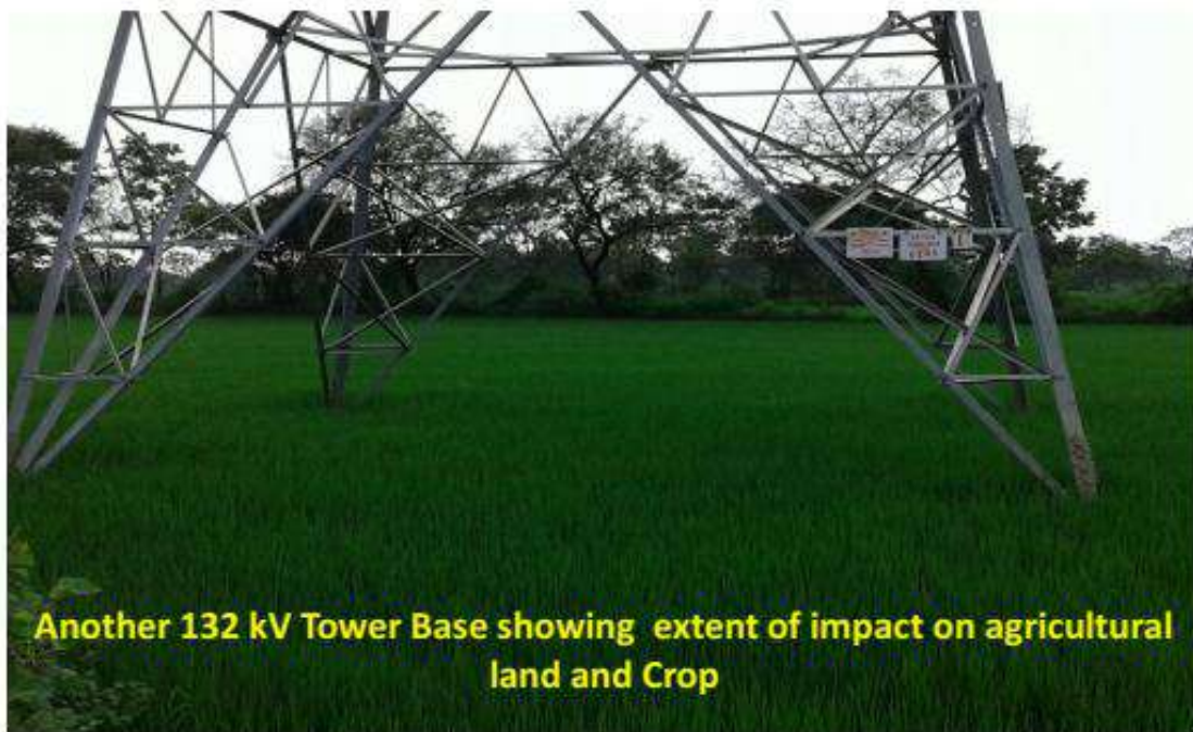
Figure 5-4: 132 kV Tower Base (TL) Showing Impact on Agricultural Land and Crop
