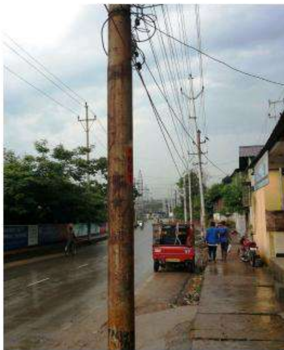
33 kV line inside city area
