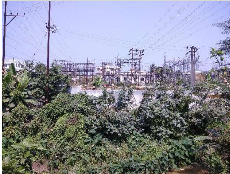
Champak Nagar Electric S/S
