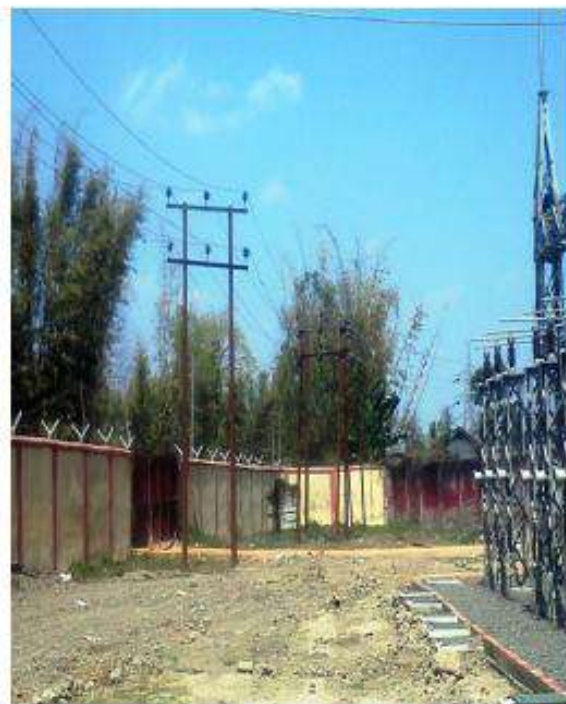
33 kV (H Pole) line inside substation
