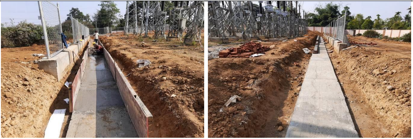
Drainage within the 132/33 kV Teok S/S
