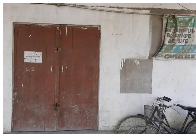
Condition of Sign Boards at 132/33 kV Sarupathar Substation
