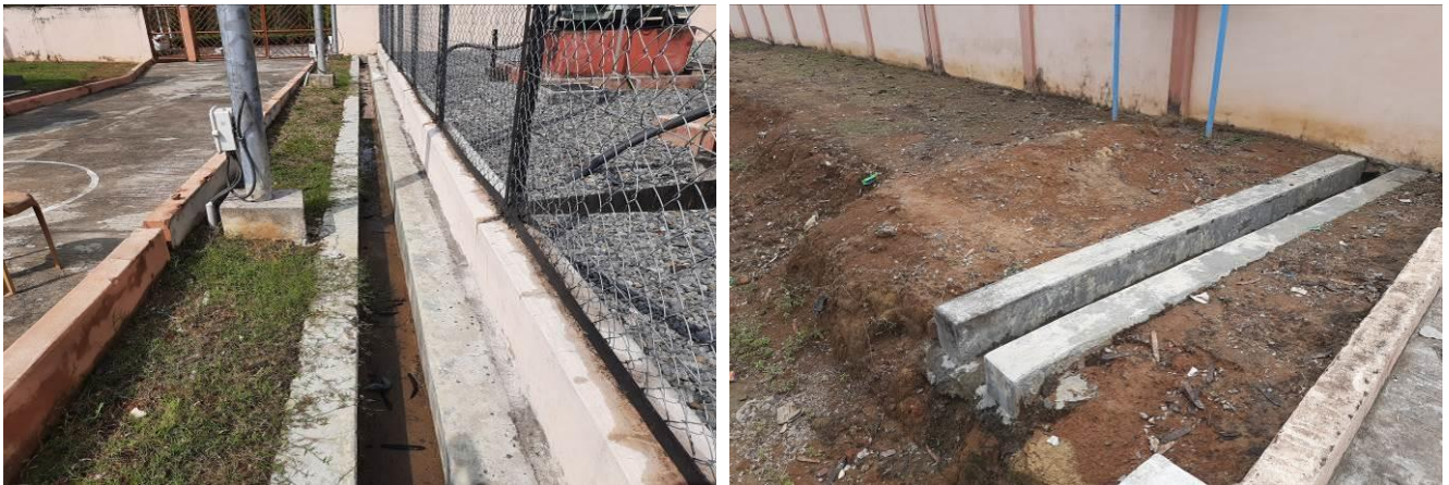
Drainage within and outside the 33/11 kV Hatimurah-II S/S
