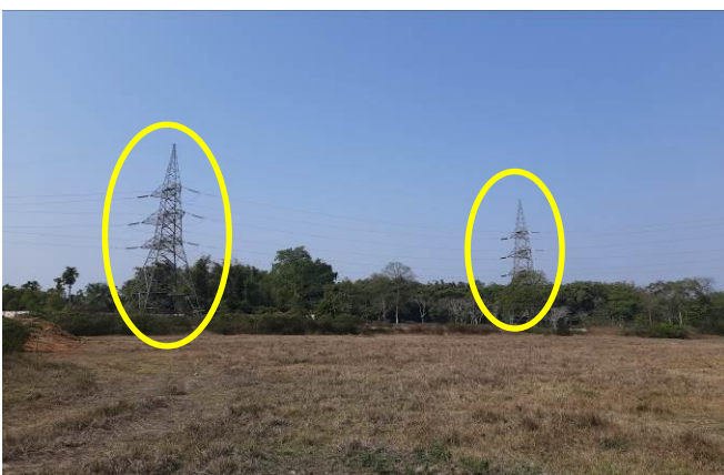
Tower No. 6/0 and 7/0
