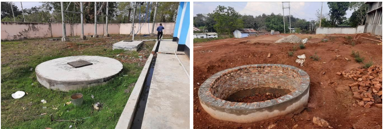
Septic Tank within the 33/11 kV Hatimurah-II and Mailu S/S
