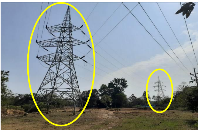
Tower No. 3/0 and 4/0
