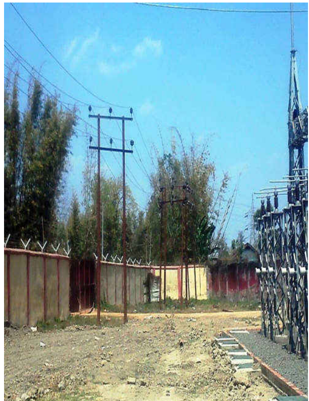
33 kV (H Pole) line inside substation
