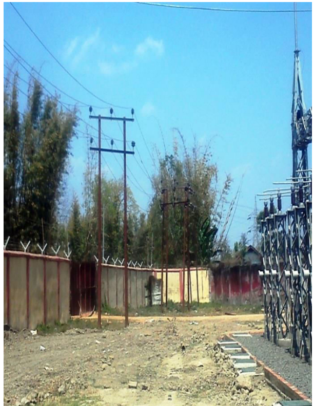
33kV (H Pole) line inside substation
