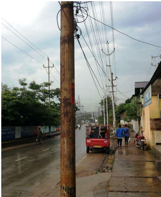
33 kV line inside city area of Assam
