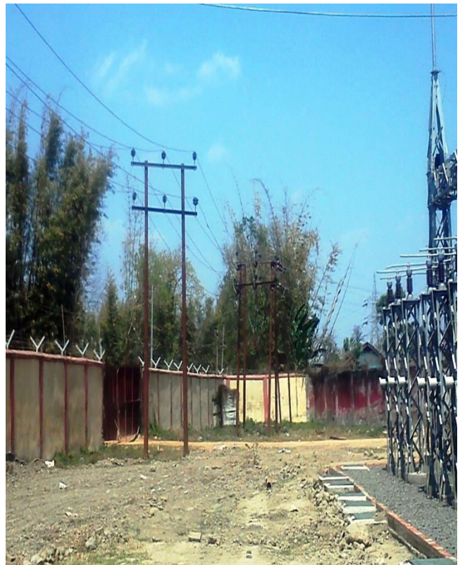
33 kV (H Pole) line inside substation
