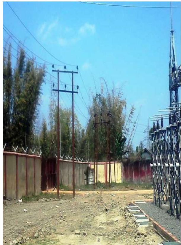
33 kV (H Pole) line inside substation
