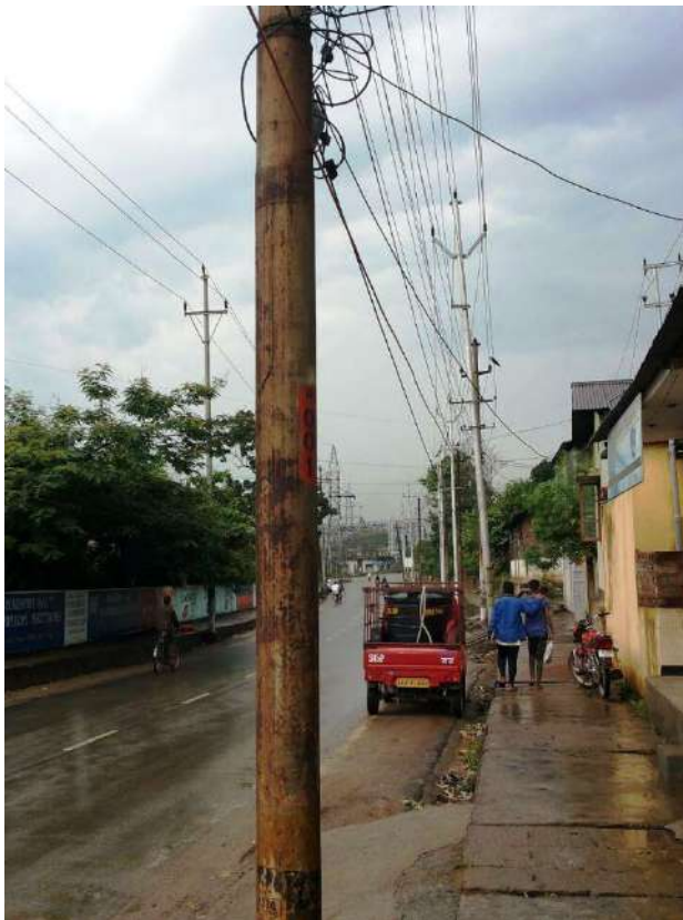
33 kV line inside city area of
