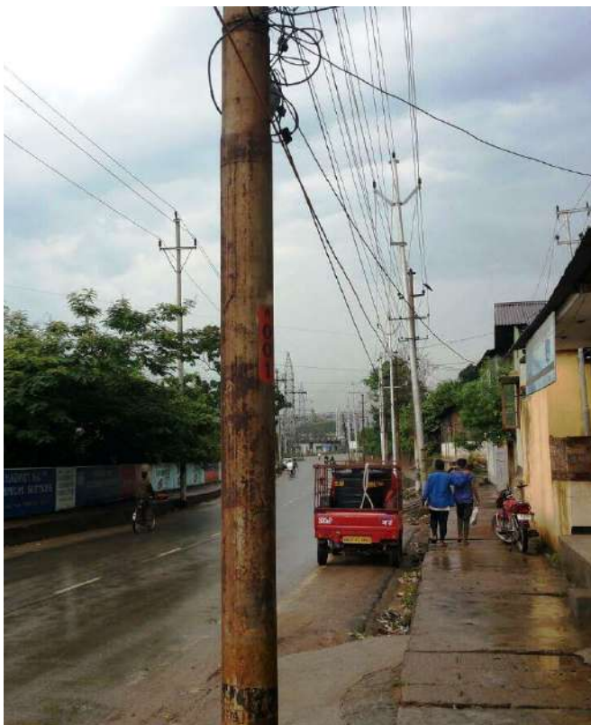
33 kV line inside city area of Assam
