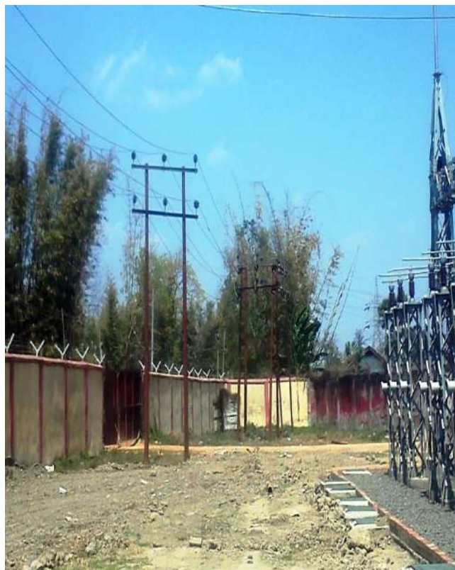
33 kV (H Pole) line inside substation
