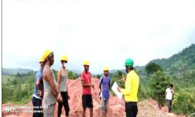
Safety briefing on Excavation, First aid, PPEs in 220 kV D/c Byrnihat-Mawngap-New Shillong
