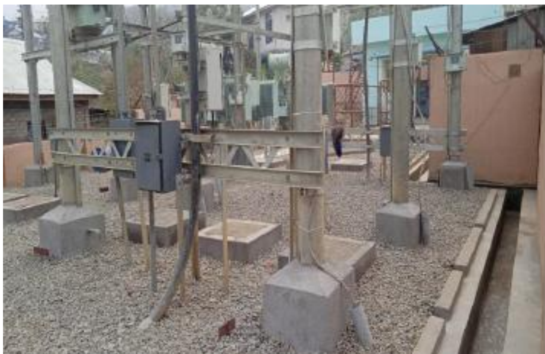
Integrated Drainage System at 33/11 Lalmati substation,
