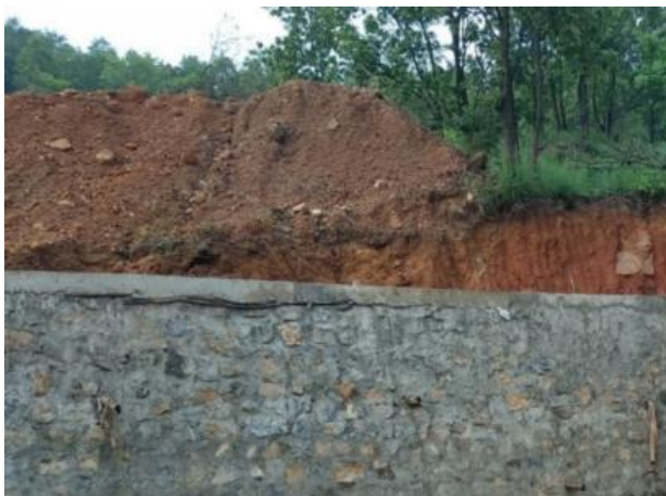
RRM wall at LILO of 132 kV MLHEP-Khliehriat Line at Mynkre
