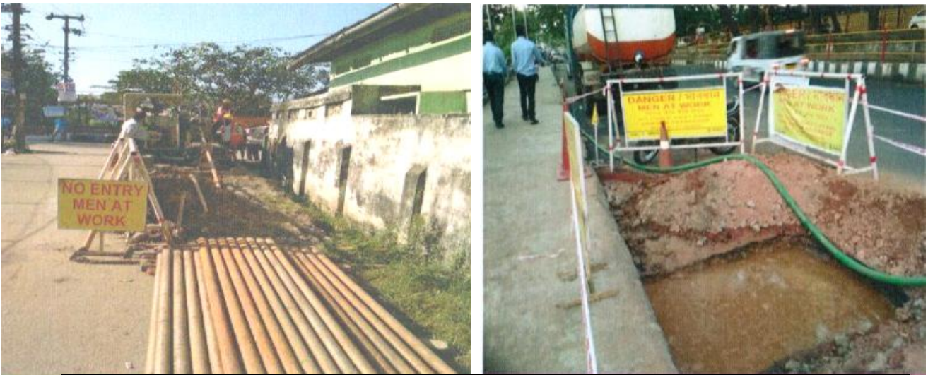
Proper Barricading of Work Area
