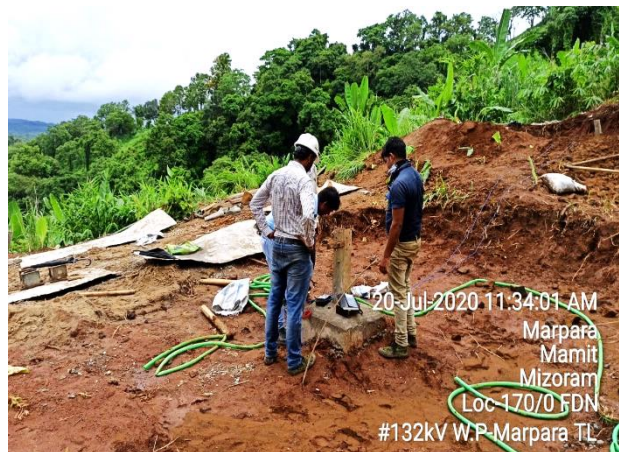
ULE Tower foundation at AP-170/0 of 132 kV 132 kV S/C West Phaileng-Marpara Line
