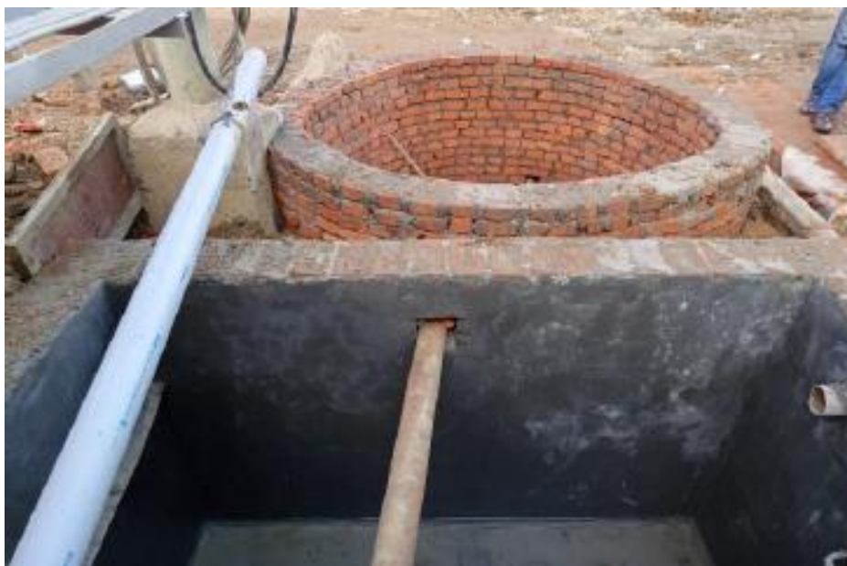
Septic Tank & Soak Pit at 33/11 Lalmati substation, Nagaland
