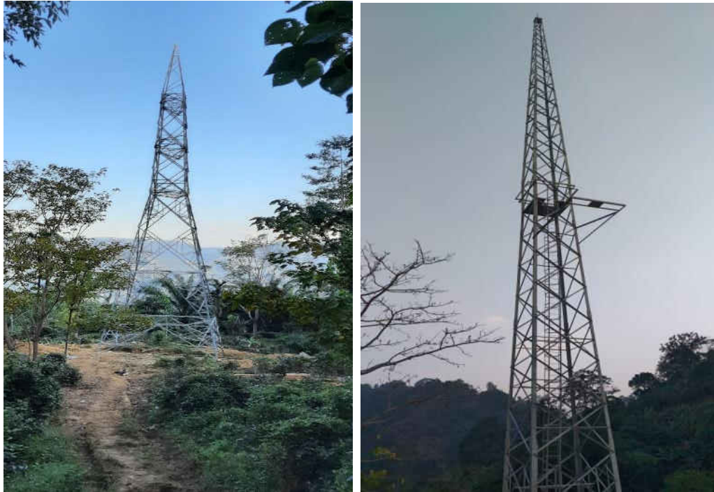
Figure 5-3 132 kV TL depicting actual position along with RoW in Undulating terrain and extent of damage
