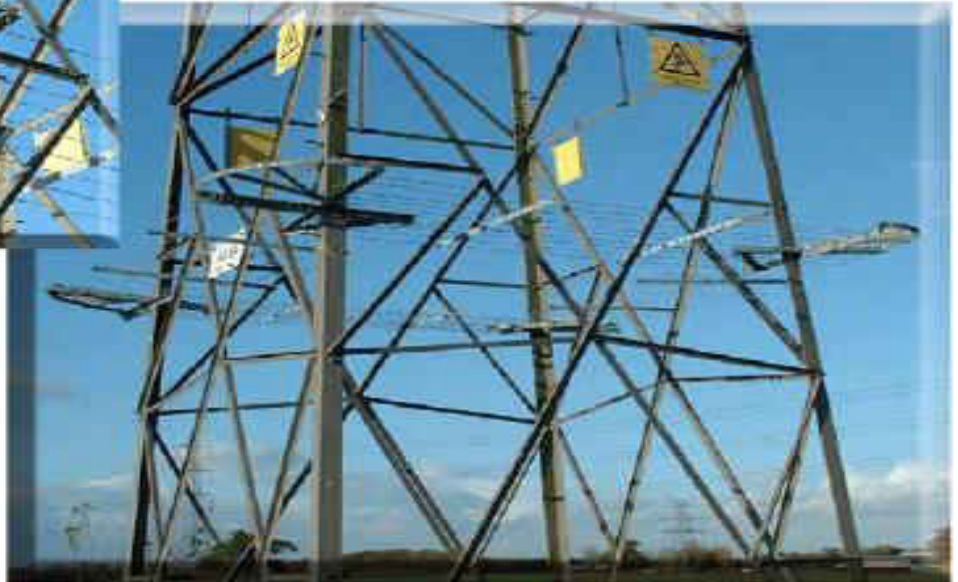
132kV TOWER ACD'S
