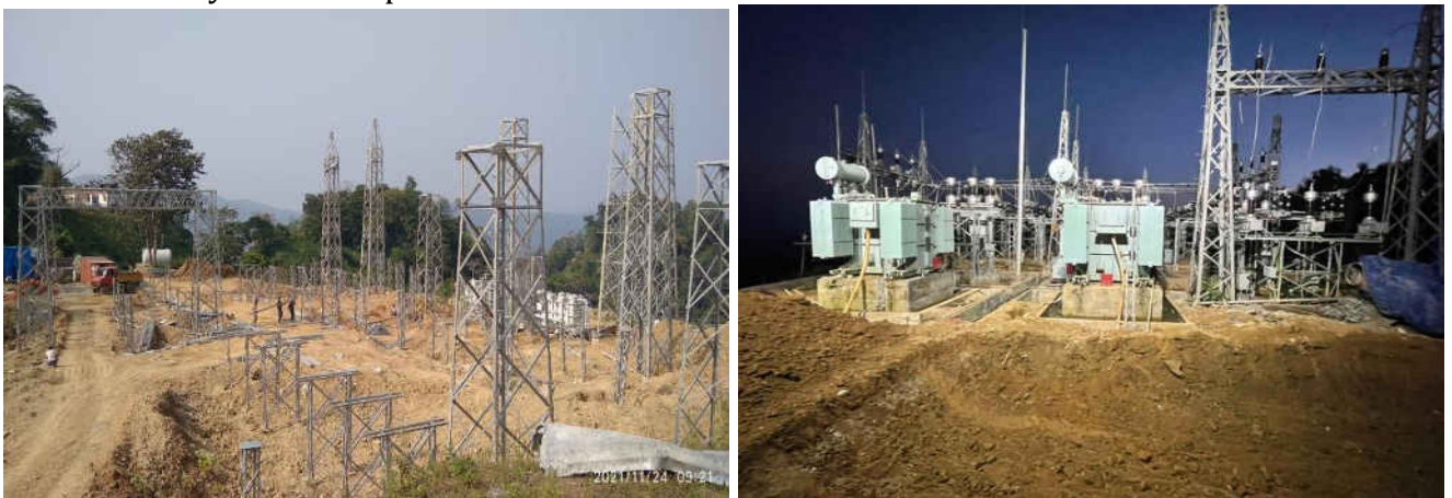
Figure 5-4 Switchyard of 132/33 kV West Phaileng S/S & Evacuation Road For construction 33/11kv
