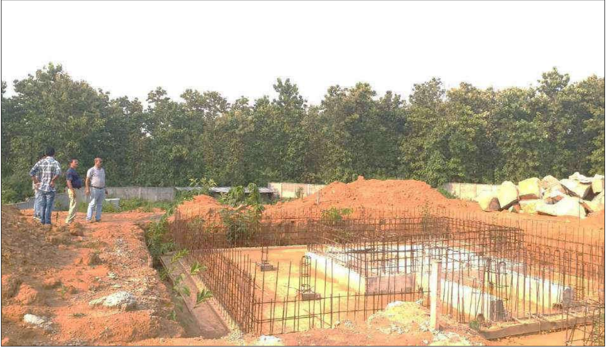
Visit to 33/1 kV Raksambre Substation
