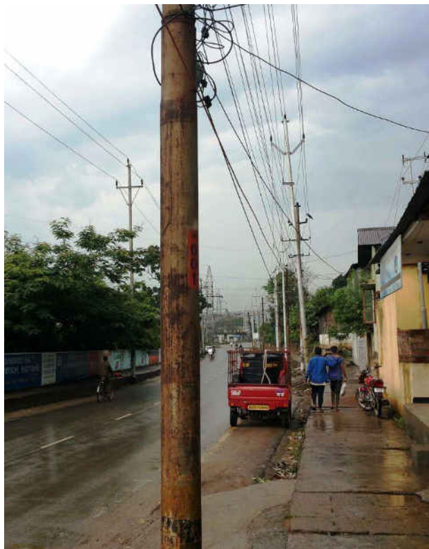
33kV line inside city area of Assam
