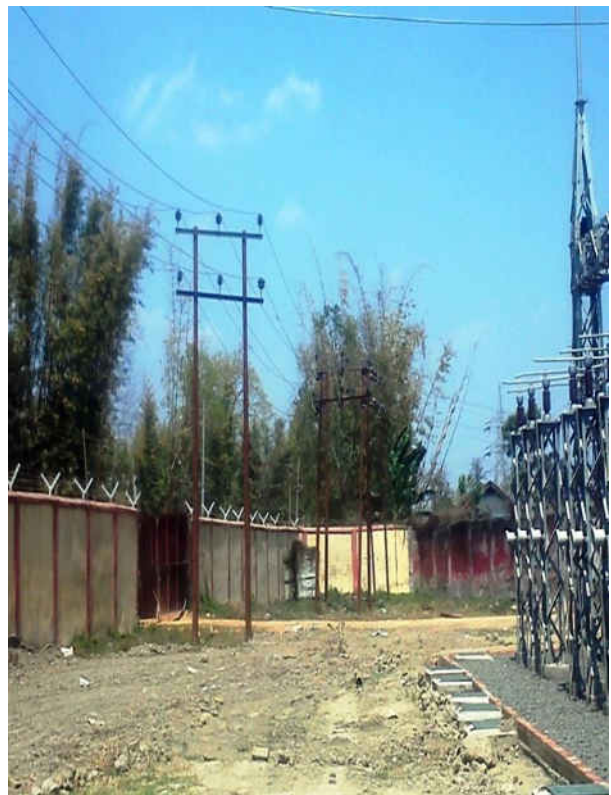
33kV (H Pole) line inside substation
