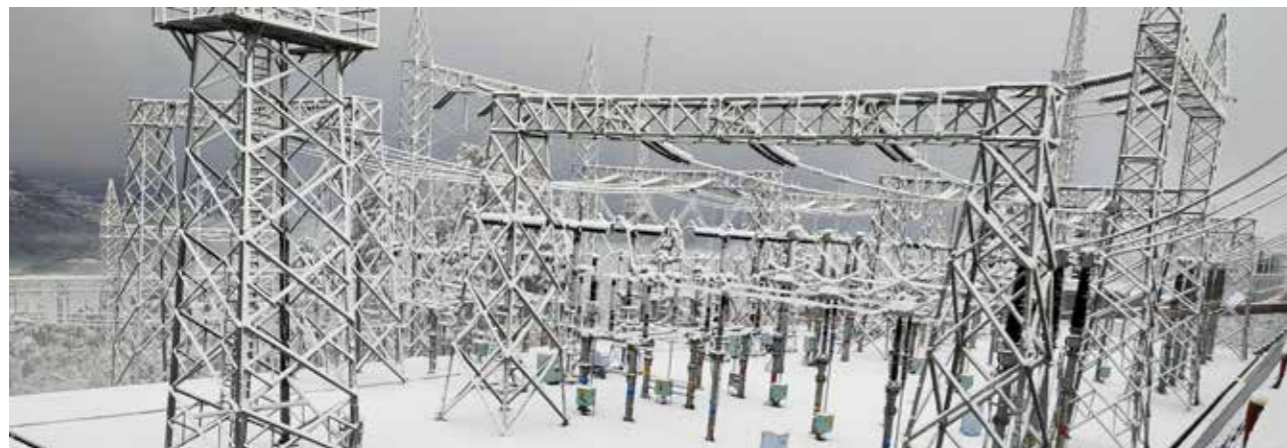
View of Pithoragarh Substation
